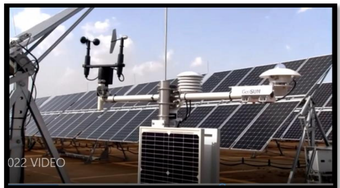
Picture 10: The Guider solar energy plant
